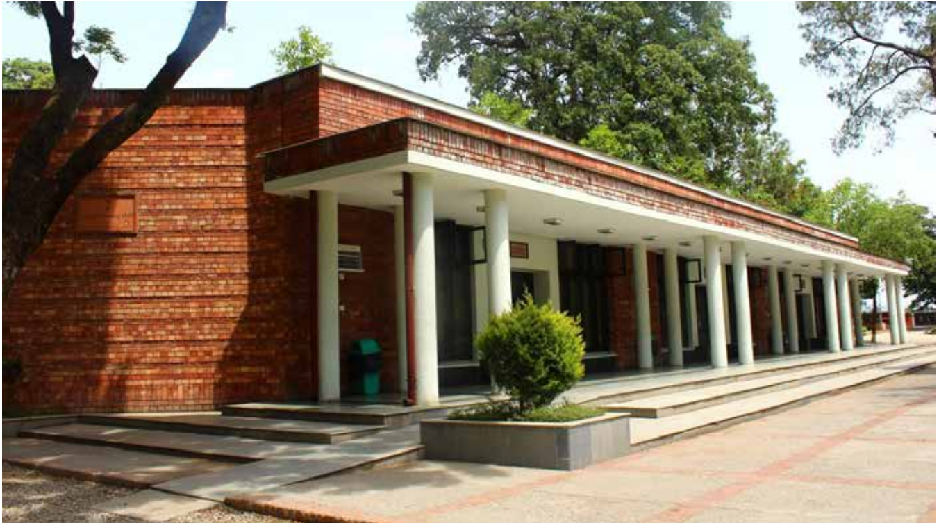
New CDH 2007- Roopak Kothari. Southern Elevation (note the white salts leached by the bricks above the sun shade, a hazard Murad Choudhary had warned against in 1995.) The columns relate to those of the Doric Order in the Hyderabad House Master's Bungalow (Fig.) but whether this is intentional or a coincidence is not known.
